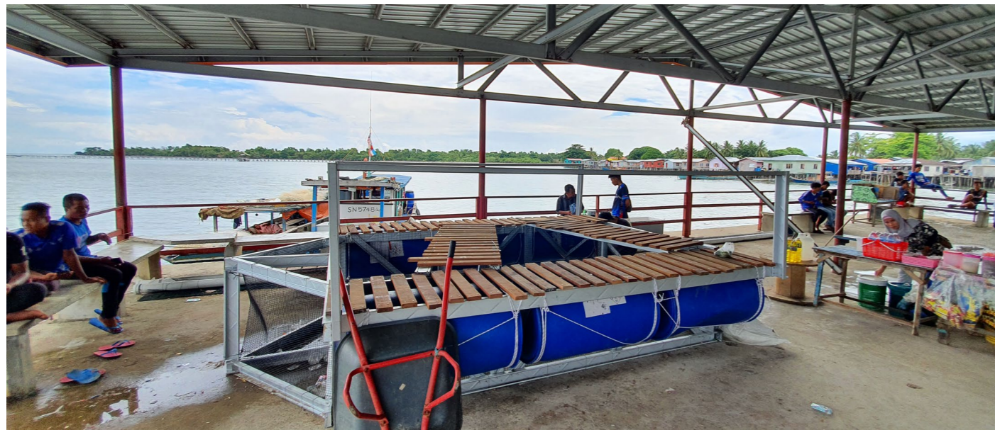
Figure 22: Construction phase of the Litter Trap in Sandakan, Malaysia
